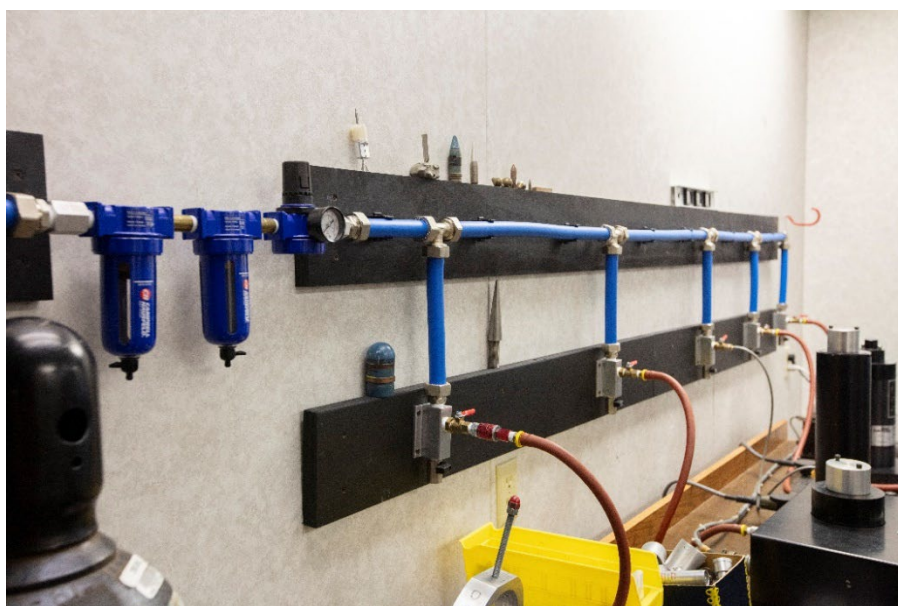
Figure 3. Pressure valve array used to supply compressed air to MOI machines.
