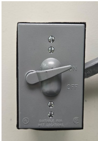
Figure 8. Switch to turn on exhaust system located toward the end of the lab by the double doors.
