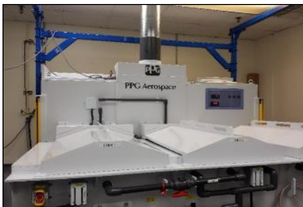
Figure 5. This anodic e-coat primer system recently installed at the USCG Aviation Logistics Center in Elizabeth City, North Carolina, was right-sized for the facility's operations after an extensive needs assessment (photo courtesy of PPG).
